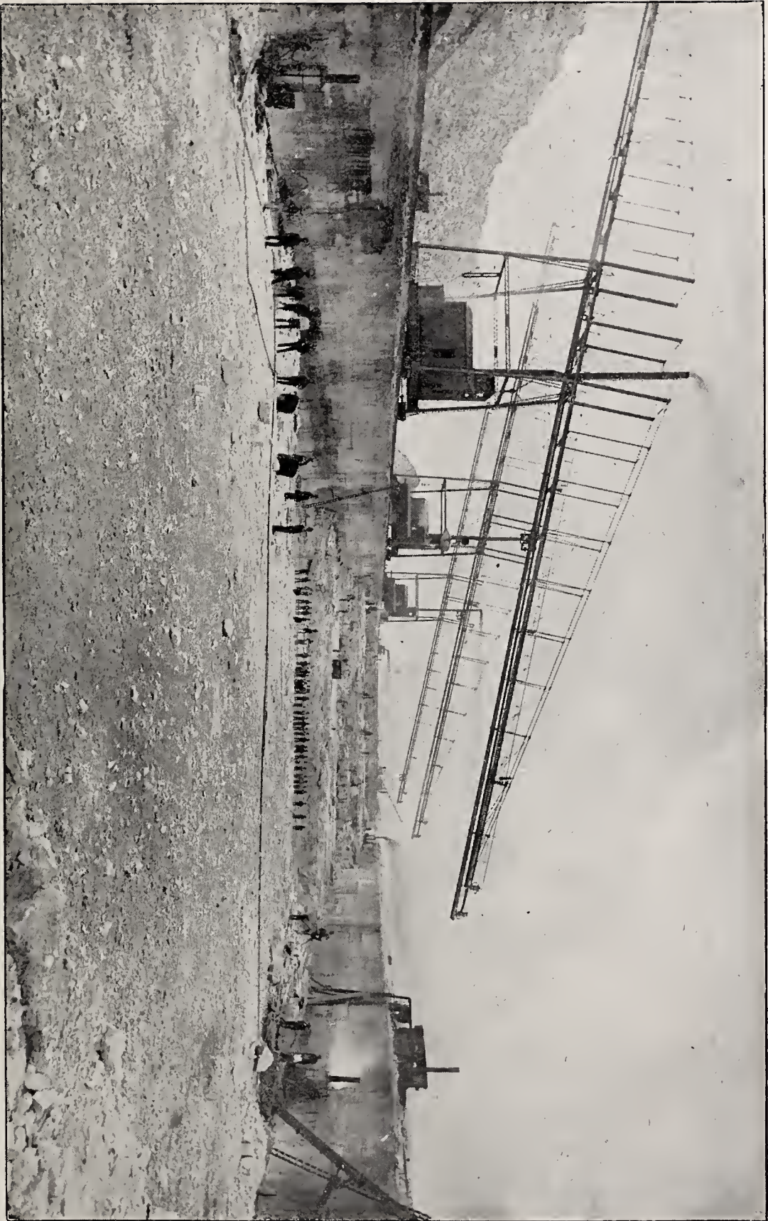
EXCAVATION IN ROCK FOR DRAINAGE CHANNEL AND WATERWAY. (FULL DEPTH IN CENTER.)
